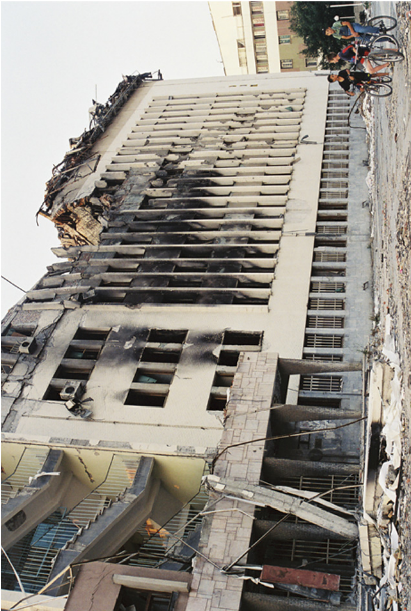
FIGURE 39 A Pristina building damaged by NATO bombings. Courtesy Lloyd Turner.
