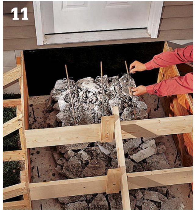
11 Lay pieces of #3 metal rebar on top of the fill at 12" intervals, and attach them to bolsters with wire to keep them from moving when the concrete is poured. Keep rebar at least 2" below the top of the forms. Mist the forms and the rubble with water.
