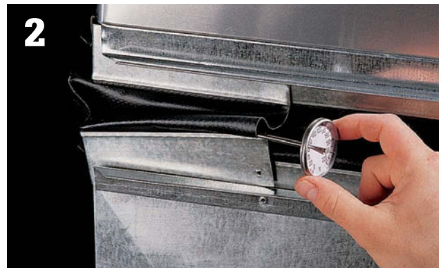
2 Check the temperature inside the supply duct and compare it with the temperature in the return duct.
