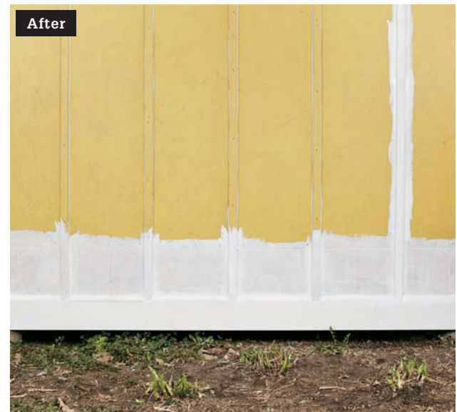
Replacing rotting siding is a common fix for wooden sheds. After painting it will look as good as new.
