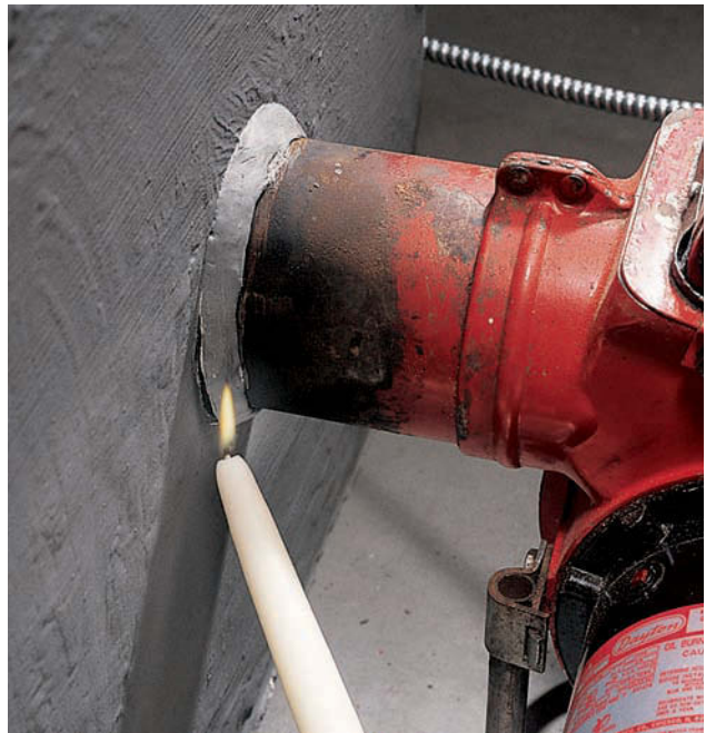
Hold a lighted candle to the joints on the flue and seams around the burner to find leaks.
