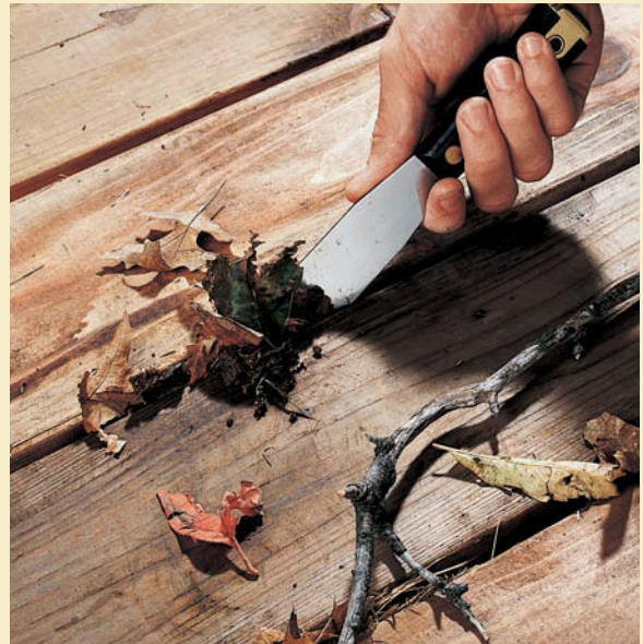
Clean debris from cracks between decking boards with a putty knife. Debris traps moisture, and can cause wood to rot.
