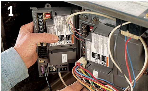
1 Remove the control center wires one at a time and switch them over to the new control center.
