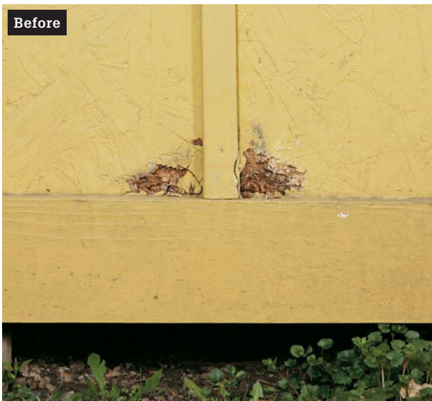
Accumulating rot defaces and devalues your shed; fortunately there's a quick fix.
