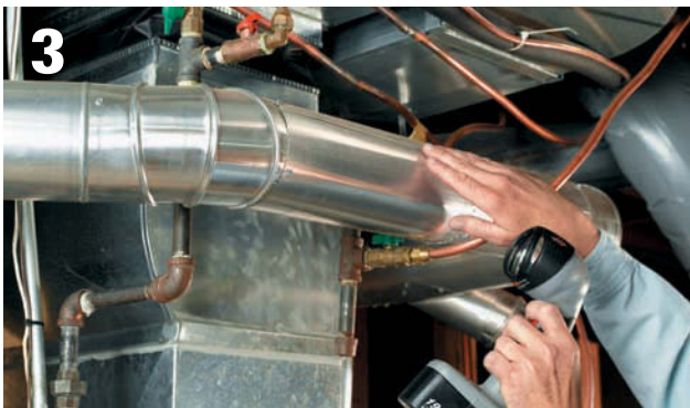
3 Inspect the areas around vent pipes for signs of corrosion. Corroded pipes will need to be replaced.
