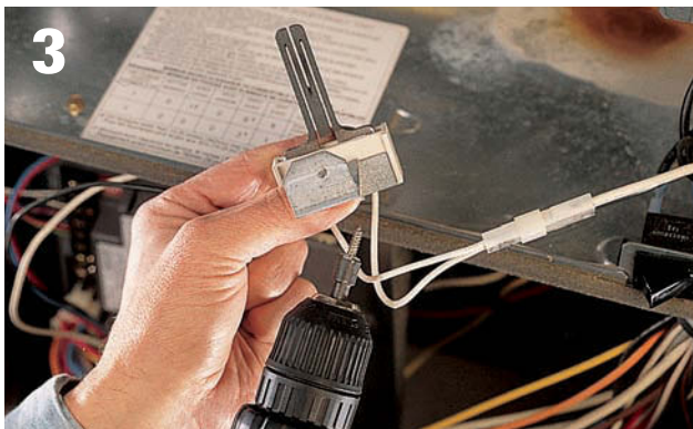
3 Disconnect the faulty hot-surface igniter from the mounting bracket.
