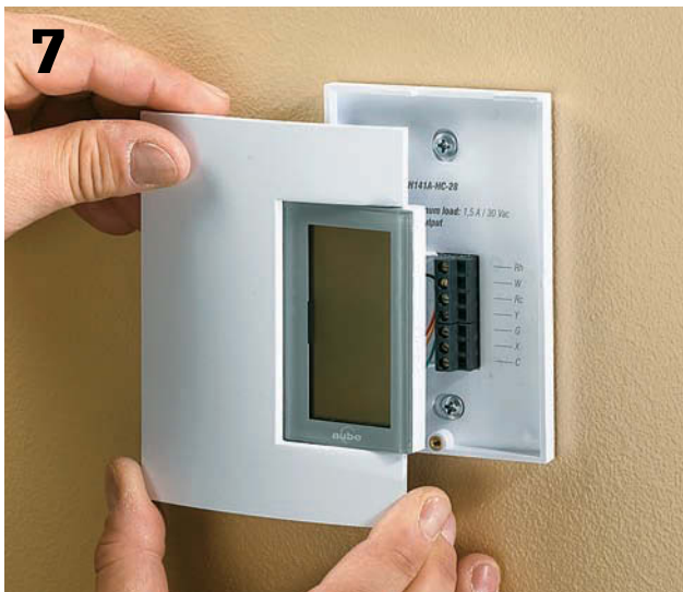
7 Programmable thermostats require batteries to store the programs so they won't disappear if the power goes out in a storm. Make sure to install batteries before you snap the thermostat cover in place. Program the new unit to fit your needs, and then turn on the power to the furnace.
