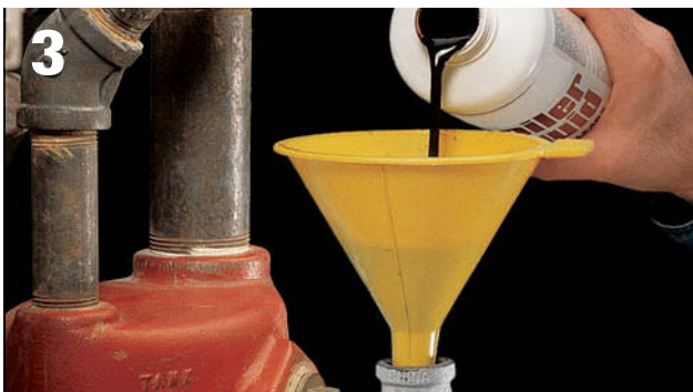
Using a funnel , add a recommended rust inhibitor to the boiler through the valve or gauge fitting.
