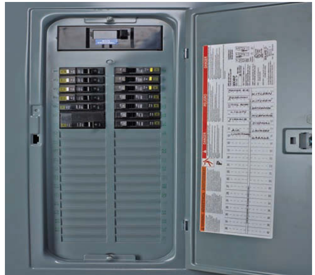
Create a circuit index and affix it to the inside of the door to your main service panel. Update it as needed.
