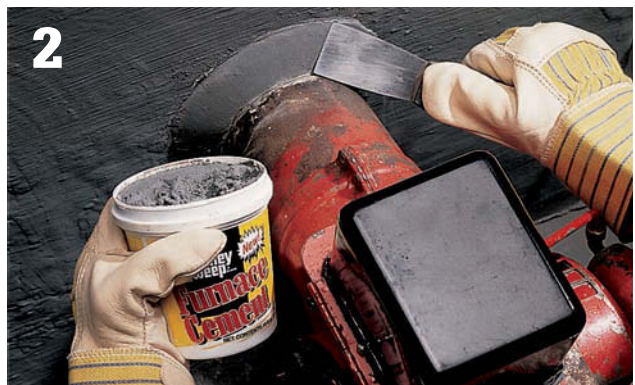
With a putty knife, apply refractory furnace cement to seal the leak.
