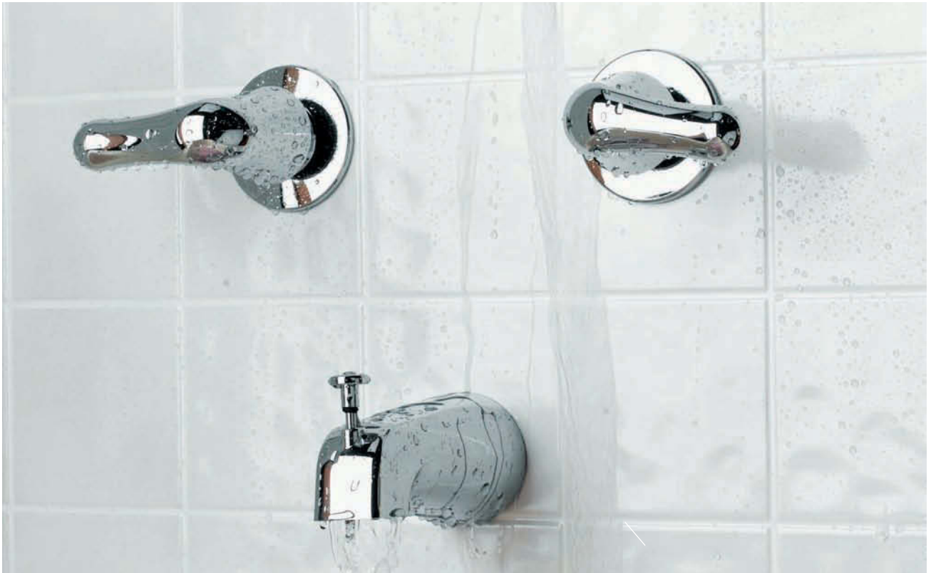
Tub/shower plumbing is notorious for developing drips from the tub spout and the showerhead. In most cases, the leak can be traced to the valves controlled by the faucet handles.
