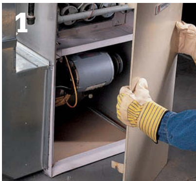
1 Remove the access panel to the blower housing and inspect the motor.
