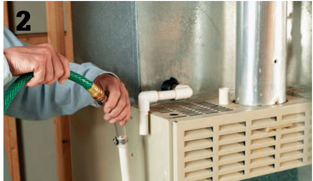
2 Clean the drain line once a year by running water through it from a garden hose.
