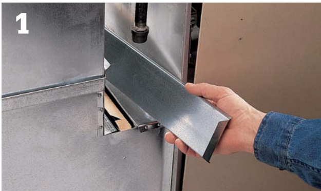
Many filters are located between the return air duct and the blower, and rest in a slot or bracket.
