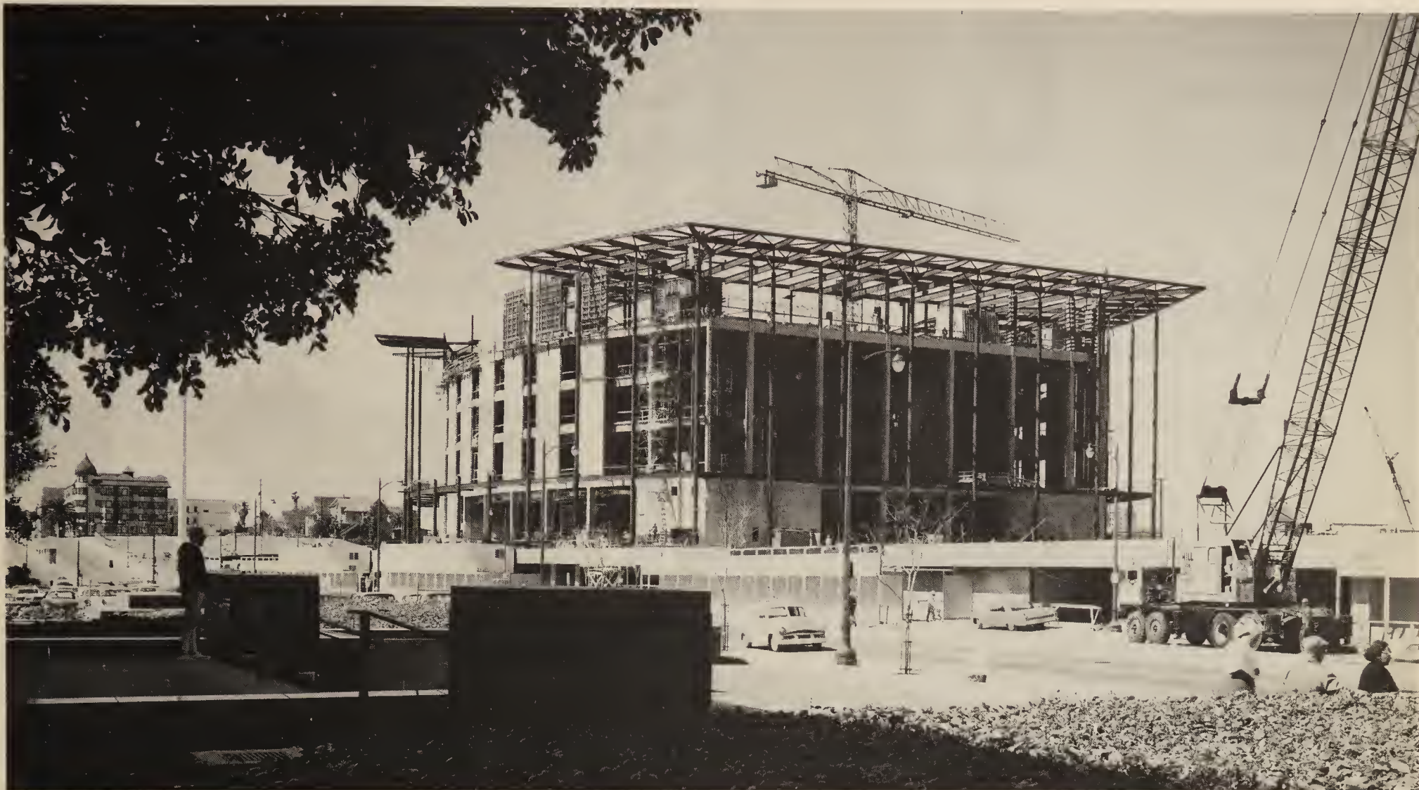
The construction of the Chandler Pavilion, Los Angeles Music Center, downtown Los Angeles, 1963.
