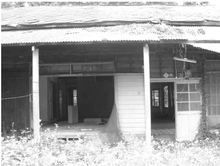
Figure 7.2 A dilapidated dormitory house at the Huwei Sugar Refinery.
