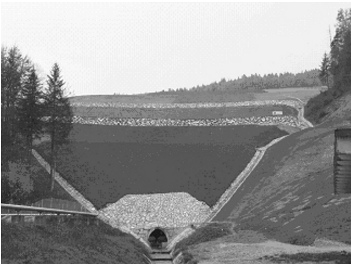
Fig.2. Jazbec pile after contouring and cover construction of the eastern slope (2007), at the bottom the outlet of the culvert draining to the Brebovčica creek.
