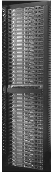
Figure D.19 The TB-80 VME rack from Capricorn Systems used by the Internet Archive. All cables, switches, and displays are accessible from the front side, and the back side is used only for airflow. This allows two racks to be placed back-to-back, which reduces the floor space demands in machine rooms.
