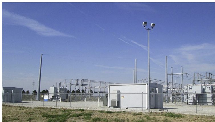
Figure 6.24 An on-site substation.
