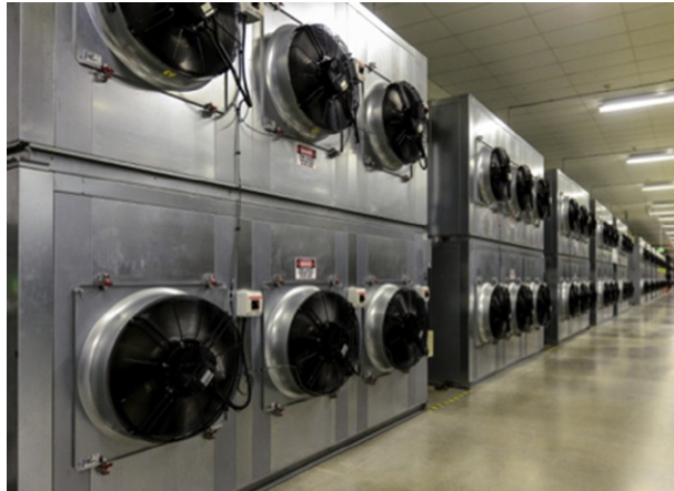
Figure 6.28 The cool air blows into the room containing the aisles of servers. The hot air goes through large vents into the ceilings where it is cooled before returning to these fans.
