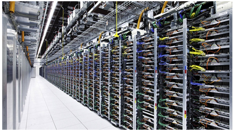
Figure 6.26 Row of servers with the copper bus ducts above that distribute 400 V to the servers. Although hard to see, they are above the shelf on the right side of the photo. It also shows a cold aisle that operators use to service the equipment.
