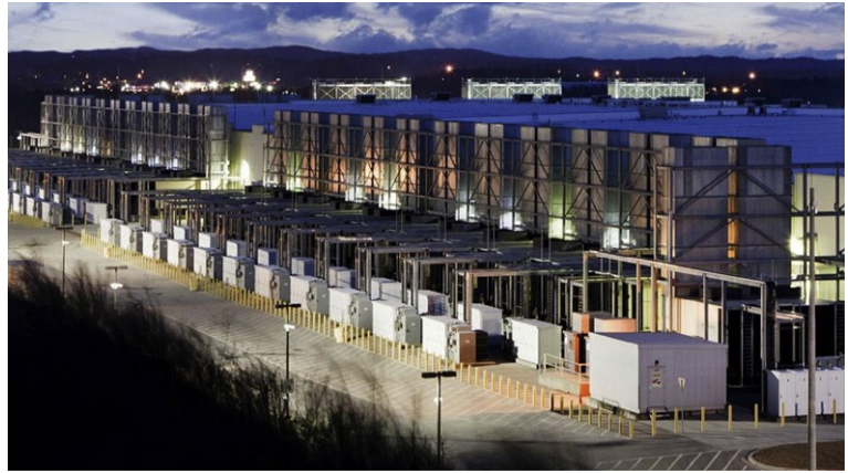
Figure 6.25 This image shows transformers, switch gear, and generators in close proximity to a WSC.
