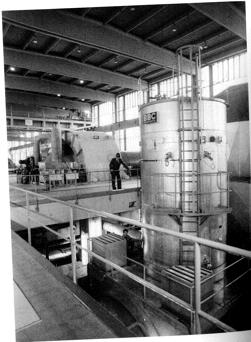
Fig. 11-3: Machine room of the 120 MW Combined-cycle Plant at Korneuburg
