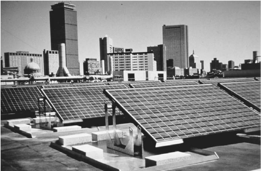
FIGURE 13-2 18 kW grid-connected pv system on the Northeastern University Student Center in Boston, MA. (Source: ASE Americas, Billerica, Massachusetts. With permission.)
