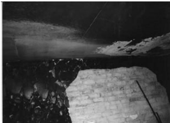
Figure 1 Plaster spalled from a wall as a result of cooling by fire fighting jets. The direction of the spray can be seen from displaced soot on the ceiling.
