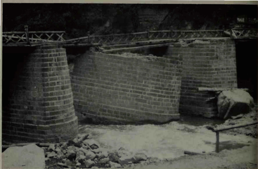
A bridge washed out by swift water.
