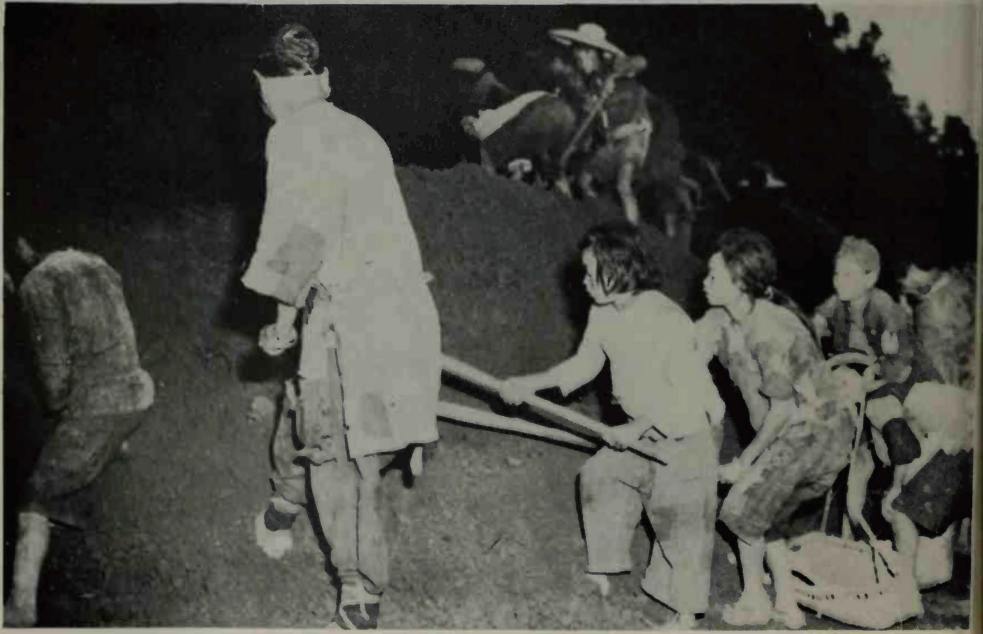
Children helping to remove a landslide.
