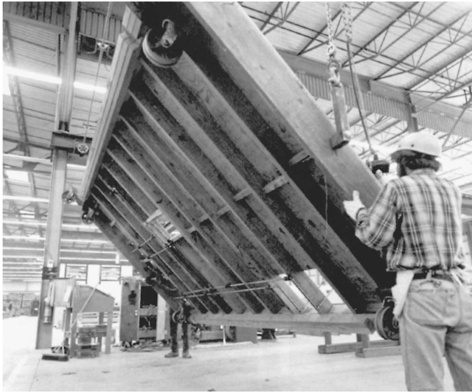
Fig. 18-15 Lifting a floor section and turning it over for subflooring and finish flooring. (Western Wood Products.)
