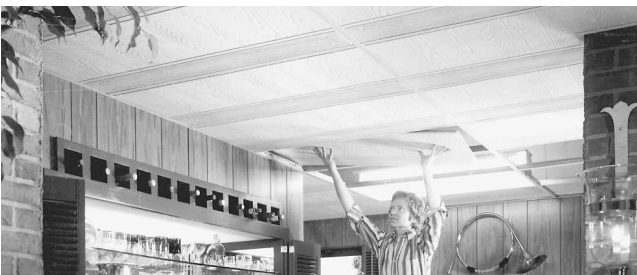
Fig. 14-55 Last, the panels are laid in place. The pattern of the tile helps to disguise the grid. (Armstrong Cork.)
