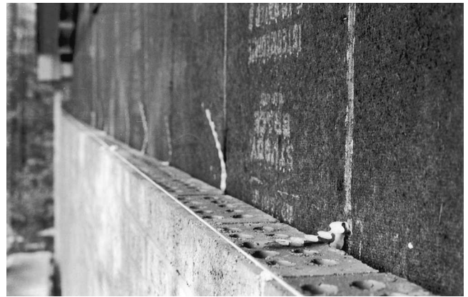
Fig. 10-65 Ties help to hold brick or stone to the wall. They are nailed to studs and embedded in the mortar.
