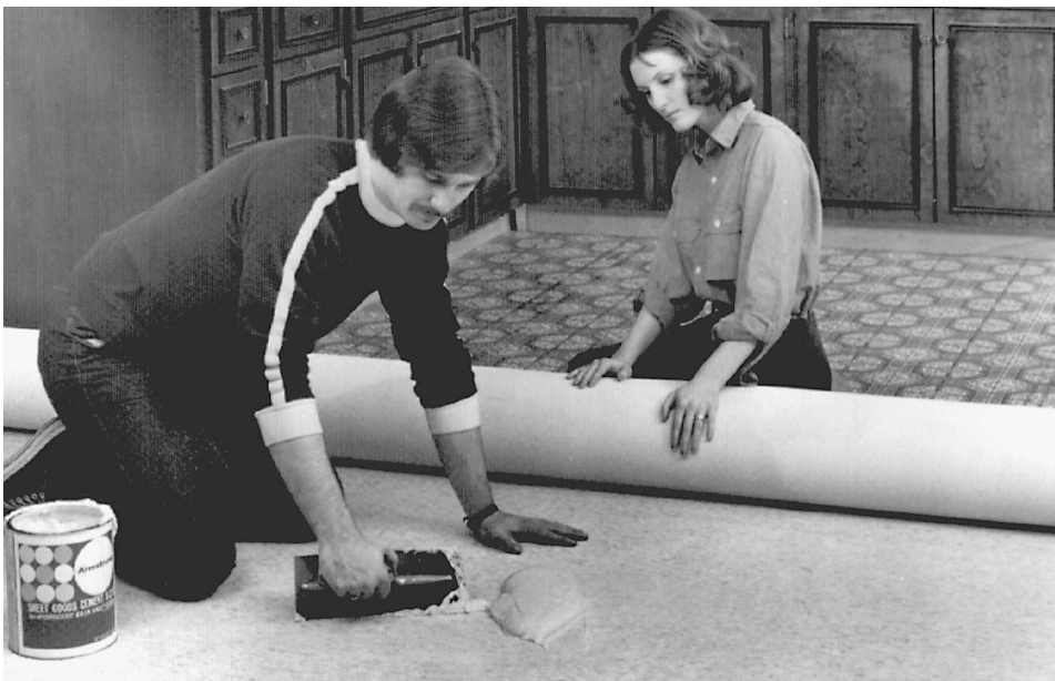
Fig. 17-46 Spread the adhesive on half the floor, and place the flooring material down. Then do the other half. (Armstrong Cork.)
