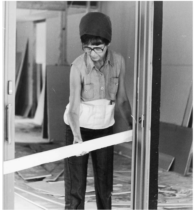
Fig. 9-142 Positioning the stationary door panel in the outer run by using a 2 × 4 wedge.
