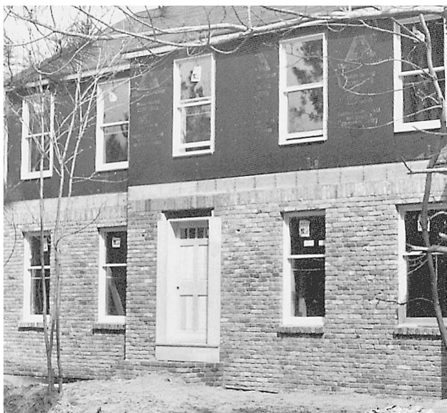
Fig. 9-14 Double-hung windows in masonry (bottom floor) and set for conventional sliding (top floor).
