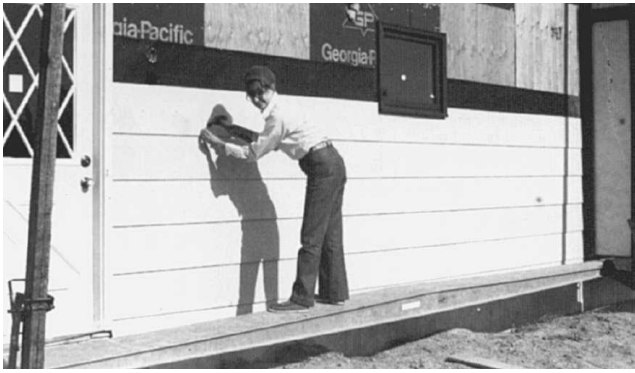
Fig. 10-8 Pump-jack scaffold for light, low work such as brick-laying, painting, and the application of siding.
