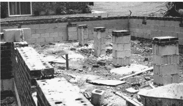
Fig. 1-46 The columns and foundation walls will help to support the floor parts.
