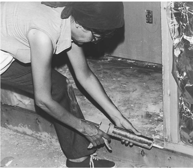
Fig. 9-136 Running a bead of caulking to seal the sill and door for a sliding door.
