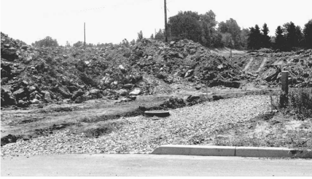
Fig. 1-44 Dirt from the basement excavation is piled high around a building site.
