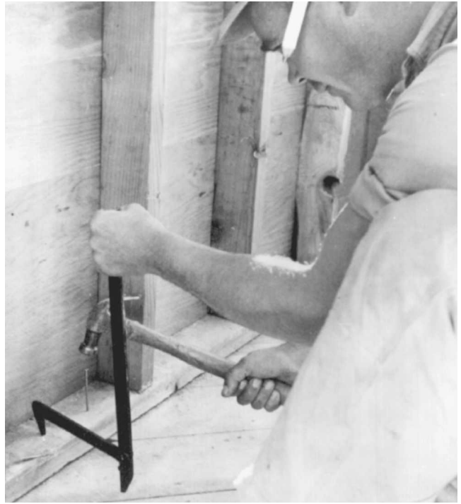
Fig. 6-40 Once the walls have been pulled into place, they are nailed to the subfloor.
