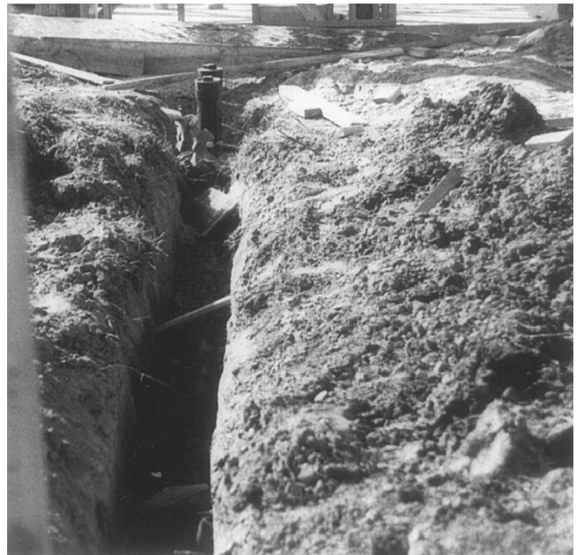
Fig. 4-12 Trenches for drains and sewers are also excavated. Clean-out plugs are usually outside the slab.
