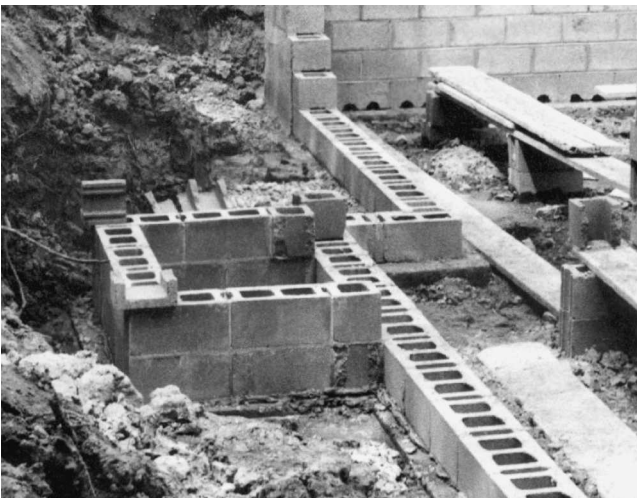
Fig. 3-10 A special footing is used for fireplaces. It supports the extra weight.
