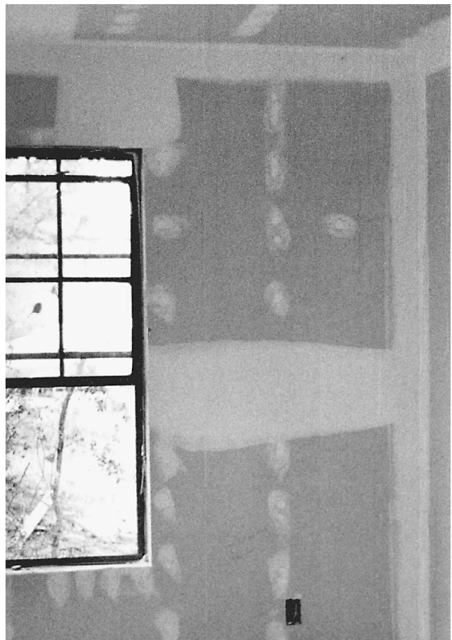
Fig. 14-6 After the Sheetrock is nailed in place, the seams and nail dimples are covered.
