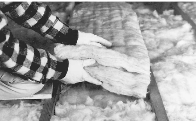
Fig. 13-15 Use insulation without a vapor barrier facing when adding to existing insulation. Batt or blankets can be laid at right angles or parallel to existing insulation. (Owens-Corning.)
