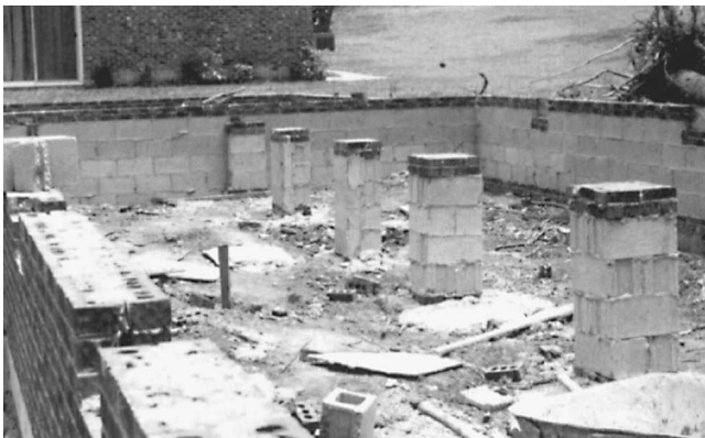
Fig. 5-4 The piers and foundation walls will help to support the floor frame.
