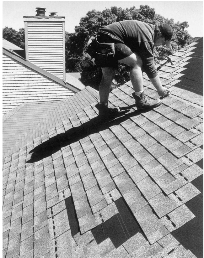
Fig. 8-36 Worker installing shingles. Note that the first strip is at the bottom. Also note the felt strip in the valley.
