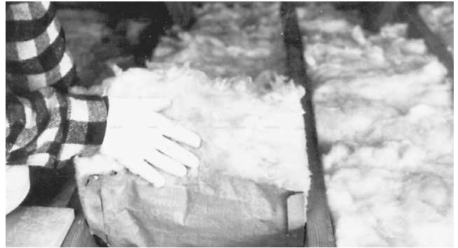
Fig. 13-17 If the attic is used for storage, the floorboards must be removed. The flooring will limit the R value to the amount of uncompressed insulation that can fit between the joists. (Owens-Corning.)
