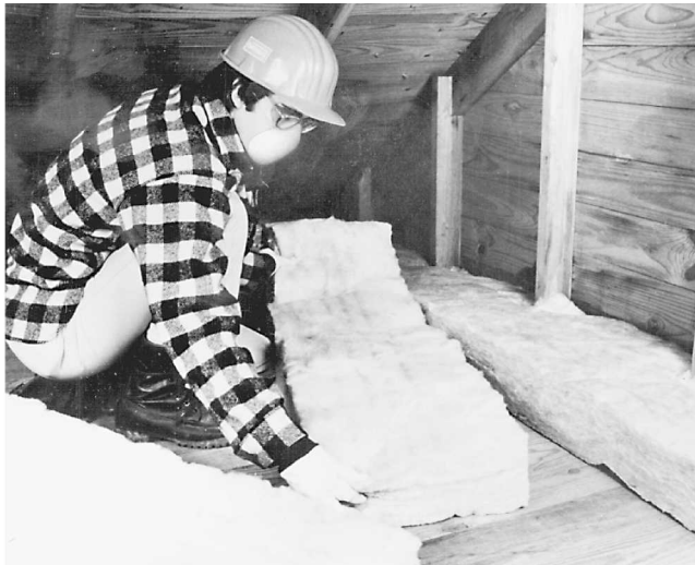
Fig. 13-14 Install insulation with a vapor barrier facing into attics with no existing insulation. The vapor barrier should face the warm-in-winter side of the structure. (Owens-Corning.)
