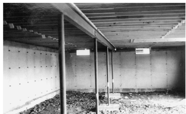
Fig. 3-8 Footings in a basement later became a part of the basement floor.
