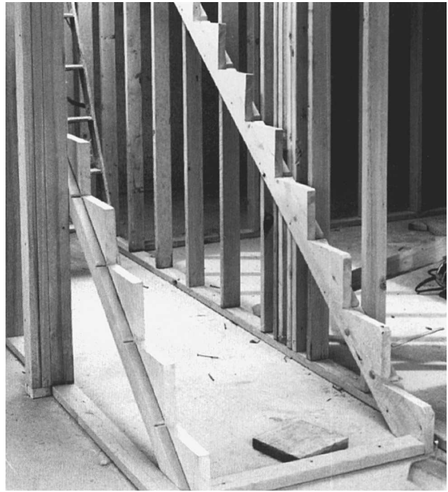
Fig. 16-1 A notched frame called a carriage is the first step in building stairs.
