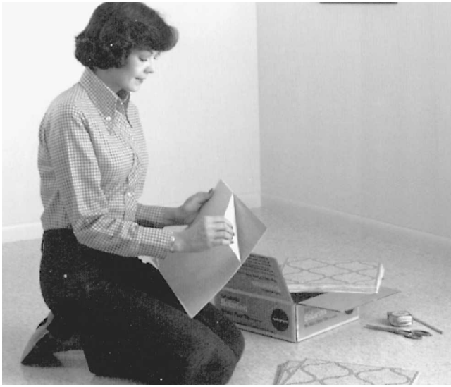
Fig. 17-47 Peel the paper off the back of a floor tile, and place the tile in a predetermined spot. (Armstrong Cork.)
