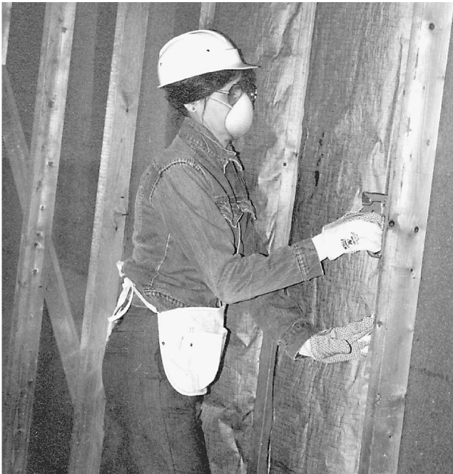
Fig. 14-1 The paper back on the insulation should face the living space. It also acts as a vapor barrier.
