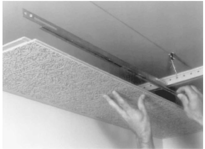
Fig. 17-66 After all the main runners are in place, begin installing ceiling tile in a corner of the room. Note how the T slides into the tile and disappears. (Armstrong Cork.)
