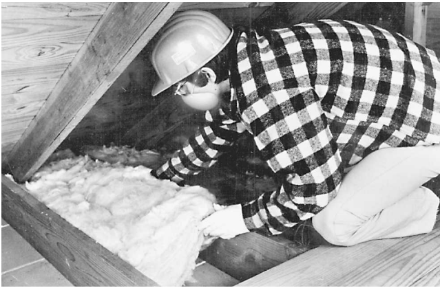
Fig. 13-19 Once the flooring has been removed, the attic should be insulated in this manner. (Owens-Corning.)
