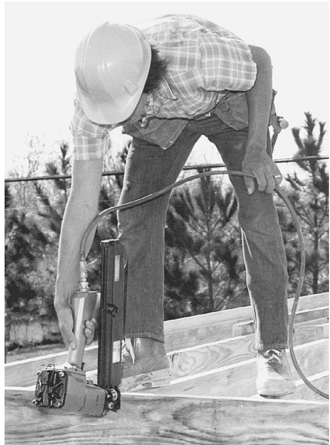
Fig. 1-1 This carpenter is using an air-driven nail driver to nail the framing members. (Duo-Fast.)
