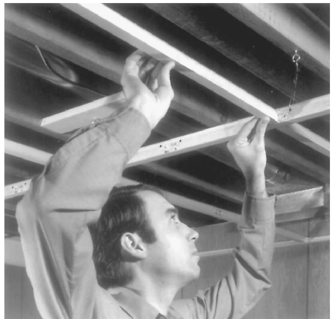
Fig. 17-67 When the main runners are in place, install cross T's between them. The T's have tabs that engage slots in the main runner to lock firmly in place. This type of suspended ceiling will have the metal showing when the job is finished. (Armstrong Cork.)
