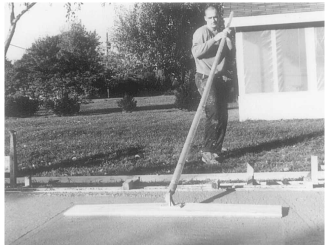
Fig. 4-23 After leveling, the surface is smoothed by floating with a bull float.
