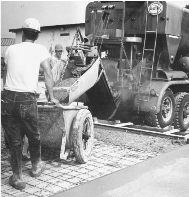
Fig. 3-21 Sometimes the concrete must be carried from the truck to the work site.
