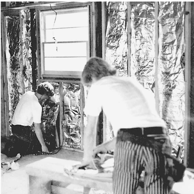
Fig. 14-2 Installing foil-backed insulation between the studs. Note that the foil is toward the living space. It is also the vapor barrier.
