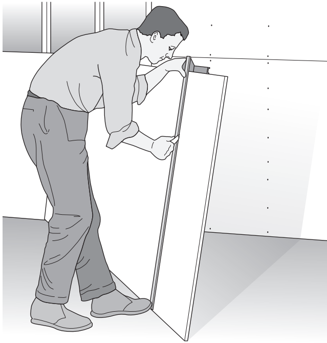
Fig. 14-16 Sheetrock is marked and scored with a knife for cutting. (Gold Bond.)
