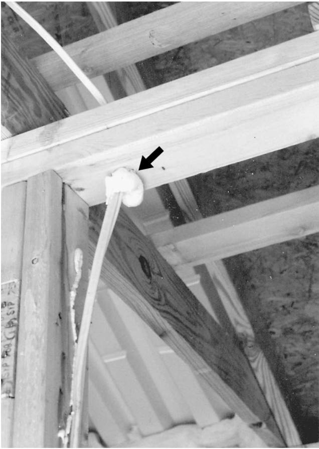
Fig. 13-62 Expandable foam used to fill the hole in an electrical wiring installation. It can serve to insulate, seal out insects, and prevent fire movement as well.
