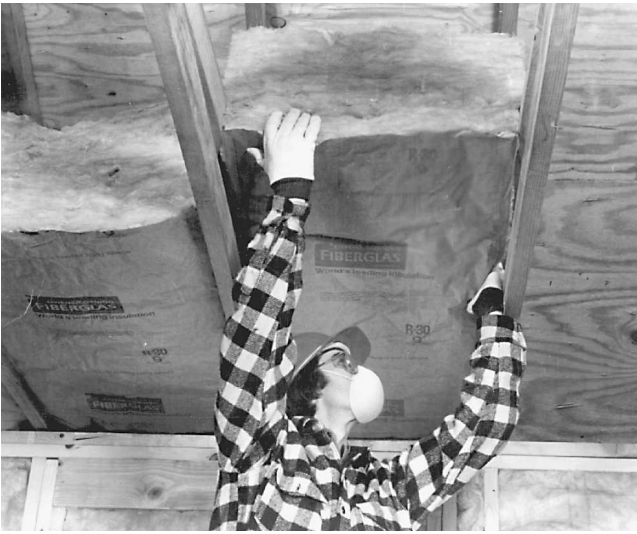
Fig. 13-13 Installing insulation in ceilings. Note the long-sleeved shirt, gloves, hat, respirator, and goggles. (Owens-Corning.)
