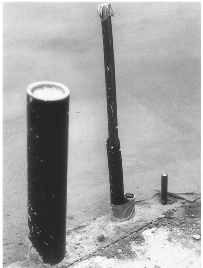
Fig. 4-10 All pipe ends are covered. This prevents them from being clogged with dirt or concrete.
