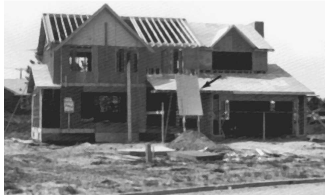
Fig. 7-96 Plywood sheathing placed on one portion of rafters. Note the ladder made for plywood lifting.
