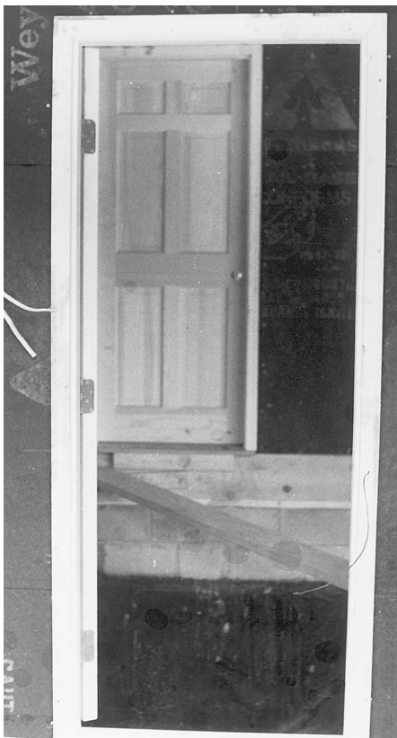
Fig. 9-85 Prehung door in place. Note the wires hanging out on the left side. They indicate where a doorbell pushbutton will go.
