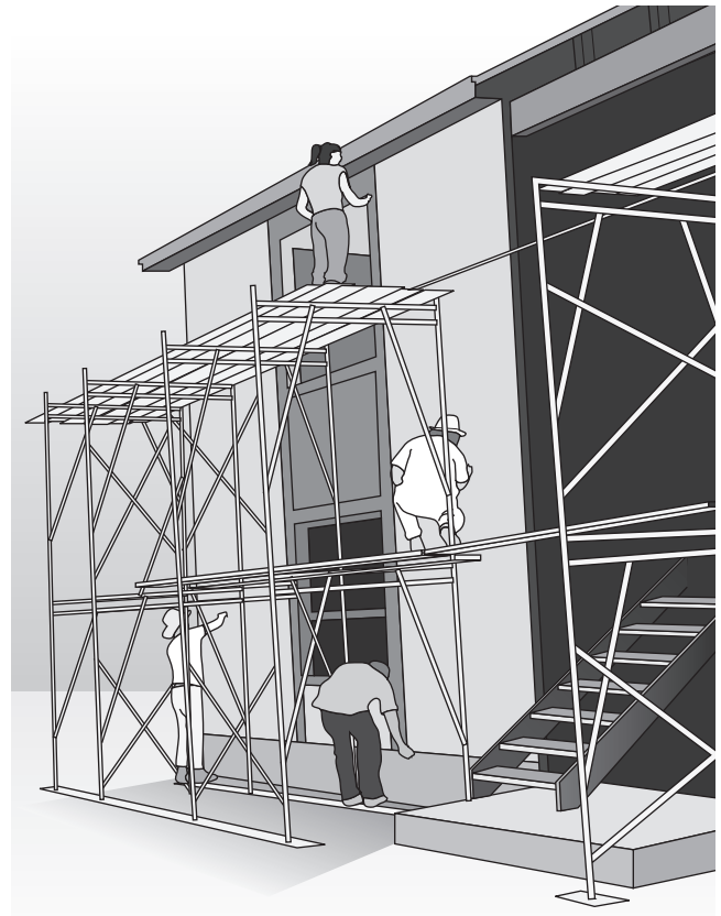
Fig. 10-14 Metal sections can be combined in several ways to get the right height and length.
