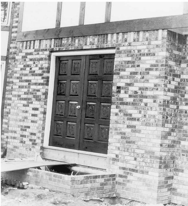
Fig. 9-87 Double doors installed. The one on the left is the active door.
