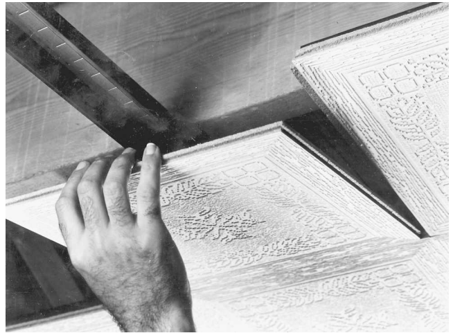
Fig. 14-56 Panels with grooved edges may be used for a system where no grid shows. (Armstrong Cork.)
