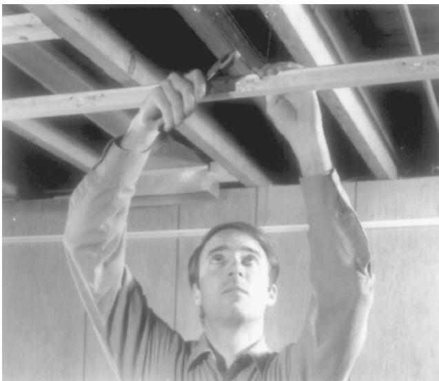
Fig. 17-65 In a basement installation, install the main runners by fastening them to hanger wires at 4-foot intervals. (Armstrong Cork.)
