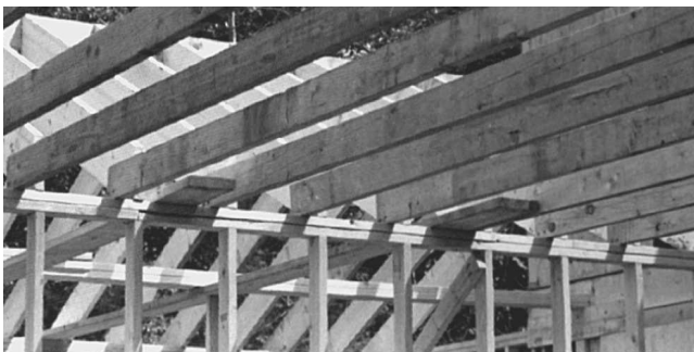
Fig. 7-83 Looking up toward the ceiling joists. Notice how these are supported on the wall plate and are not cut or tapered. Two nails are used to toenail the joists to the plate.
