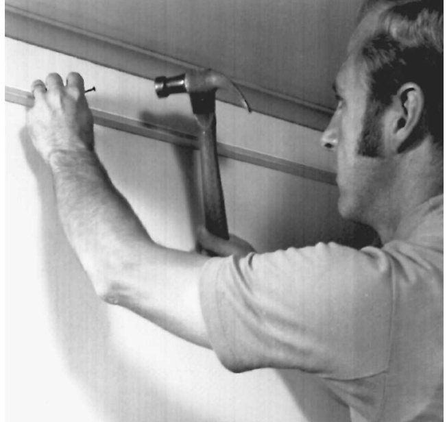
Fig. 17-62 For a new suspended ceiling, nail molding to all four walls. (Armstrong Cork.)
