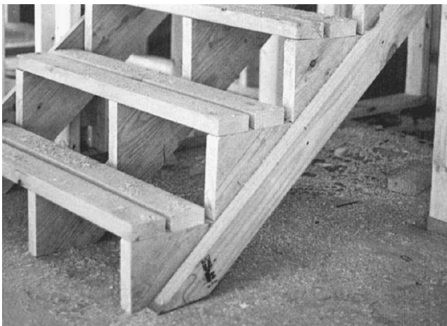
Fig. 16-7 Two-inch lumber is used for temporary steps during construction. It can be left as a base for finish treads.
