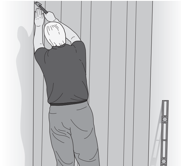
Fig. 14-37 Finally, the panels are nailed in place. A level may be used to align the panels. (Masonite.)
