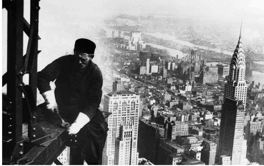
The Chrysler Building is visible (far right) behind a worker constructing the Empire State Building.
