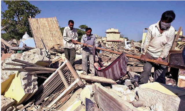
The clean-up operation begins after the devastating earthquake in Gujarat.
