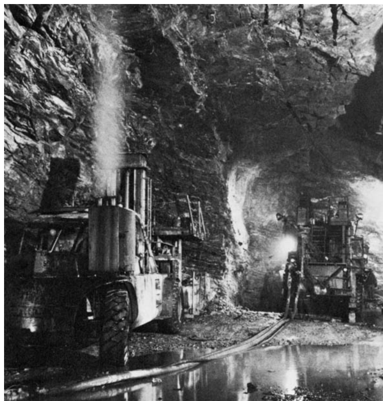
Excavation of the diversion tunnel prior to construction of the Revelstoke dam.
