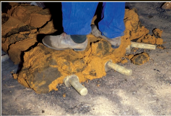
Making the motogama (base wall), including the three holes through which slag (waste) can run out during the operation of the tataru.
