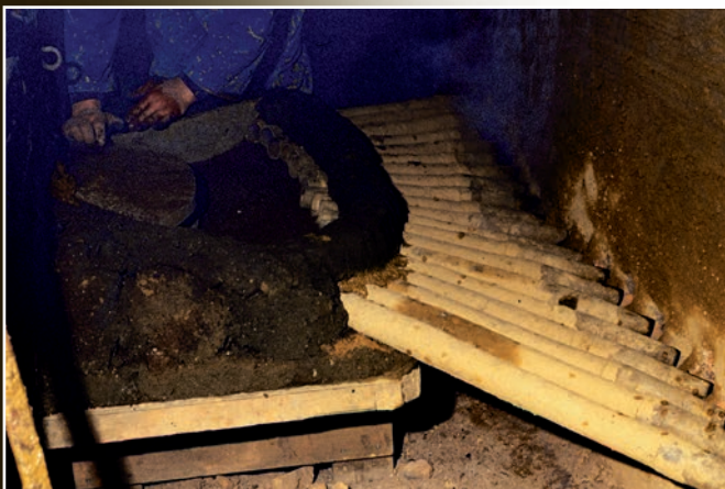
Placing bamboo pipes from the fuigo (bellows) through the furnace. These pipes will serve as ducts to inject air from the fuigo into the furnace.
