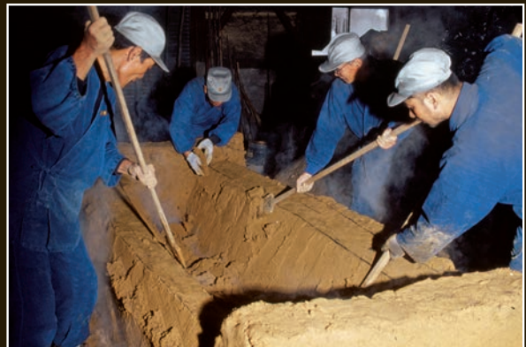
An 8-inch (20 cm) high clay wall is erected, and excess clay is shaved away.
