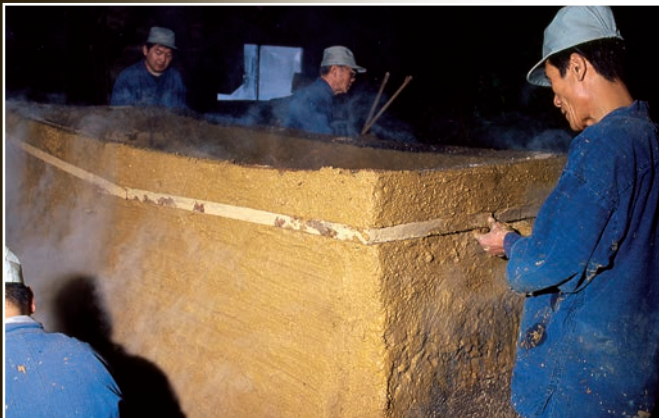
The completed furnace is reinforced with steel bands to maintain its shape during the smelting operation.
