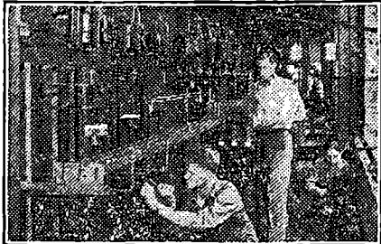
A Real Switchboard in the Coyne Shops
