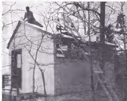
Aluminum ridge cap is nailed to roof beams as last step. Door and windows have already been installed.
