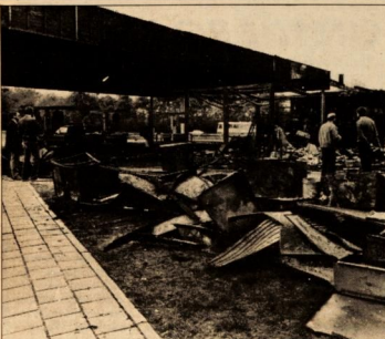
Shell Filling Station Reduced to Rubble
