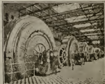
Generators in Swedish Power Plant—Note Great Size
