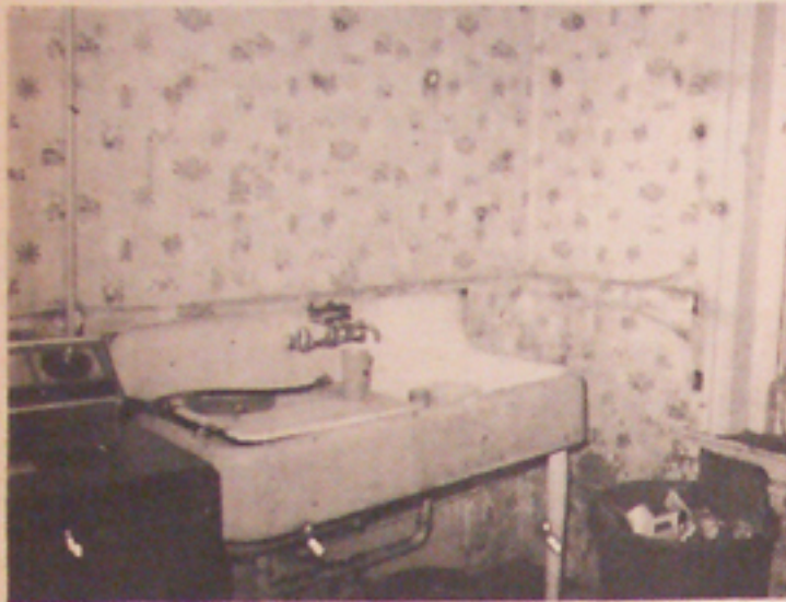
KITCHEN SINK AND PEELING WALL PAPER
