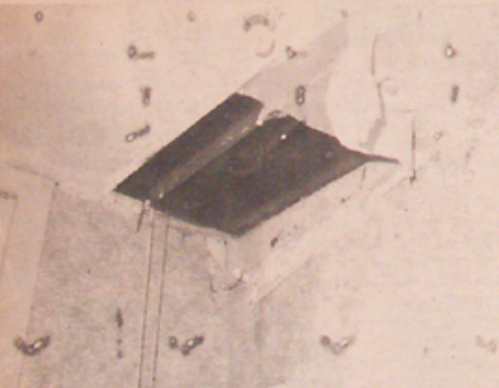
HOLE IN BATHROOM CEILING
