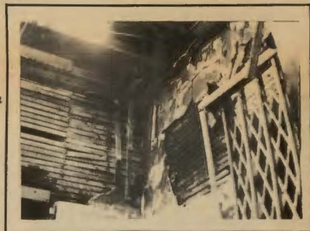
Ceiling and wall where axe was used
