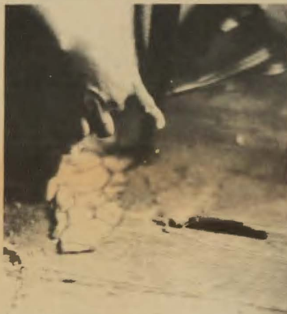
HOLES IN FLOOR OF MRS. WASHINGTON'S APARTMENT.
