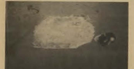
Plaster on the kitchen wall will fall out again, making it possible for the pigeons to get back into the house
