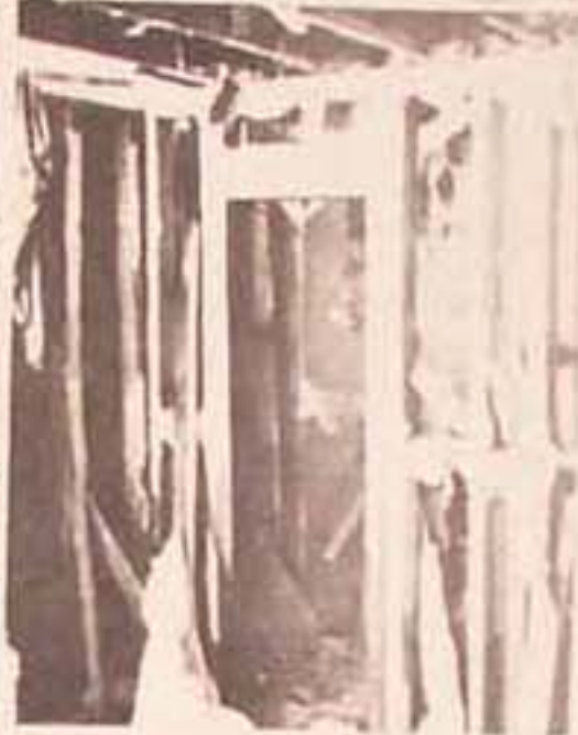
INSIDE OF DEMOLISHED HOUSE, WRECKED BY SICK SADISTIC RACISTS, CREATING VICTIMS OF BABYLONIAN TERROR.
