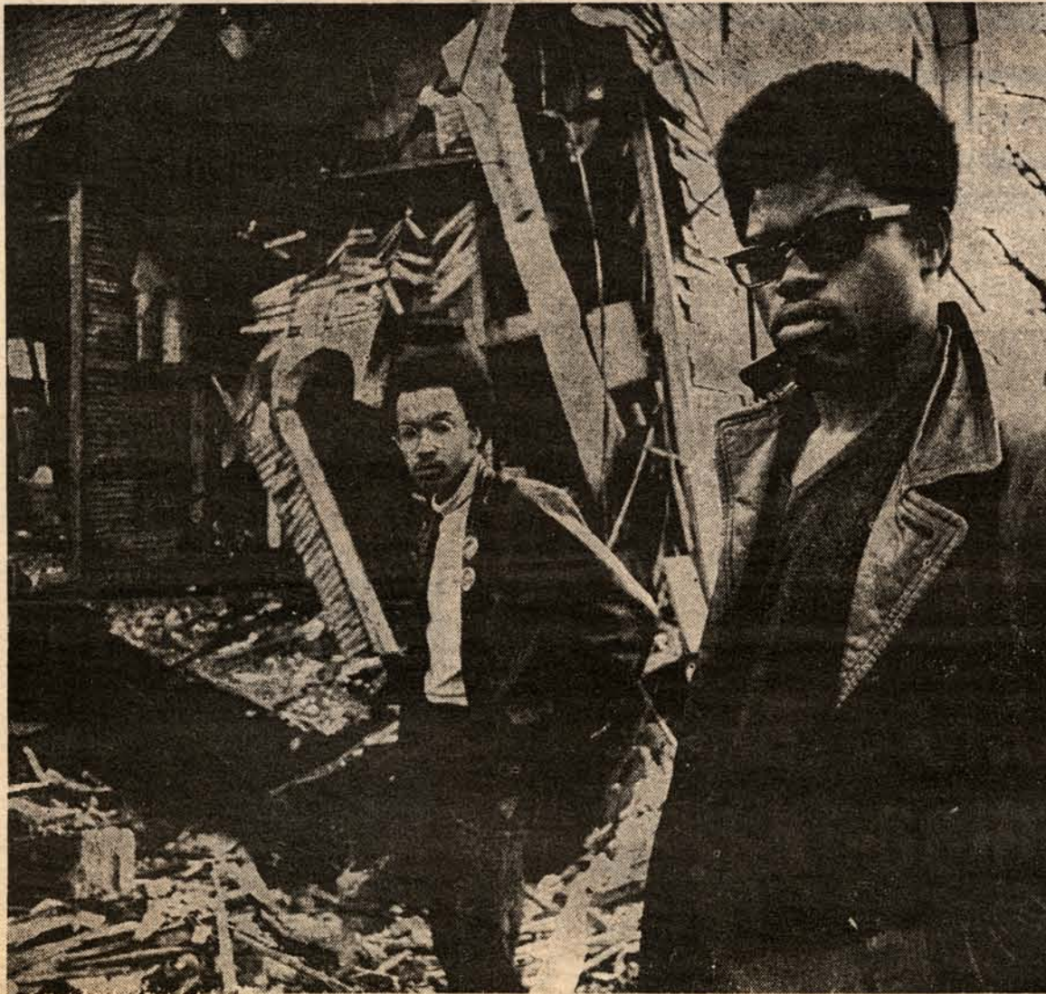
Damage is inspected by Lt. Steve Green and deputy Min. of Ed. Charles Knox
